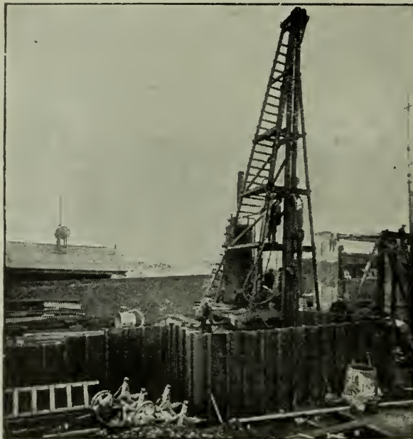
Illustration shows "Universal-Joist" Piling being Withdrawn by No. 6 McKiernan-Terry Hammer, to be redriven on the same job.
